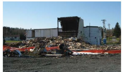
The partiality demolished fish plant in Terence Bay
